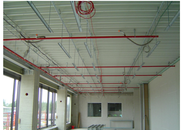
Fig. 5: For assembly, the traverses are suspended from the ceiling using threaded rods and aligned
